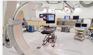
Hybrid operating room
